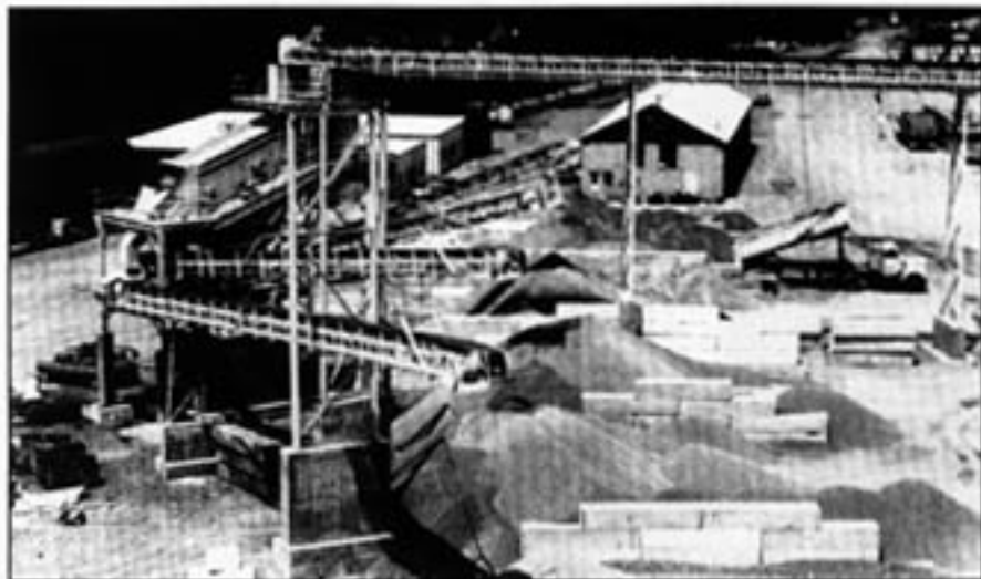
Balf produces all products directly off of its screens. Flopgates and conveyors provide flexibility without crusher and screen changes. Many unwanted products can be recycled through the plant.
